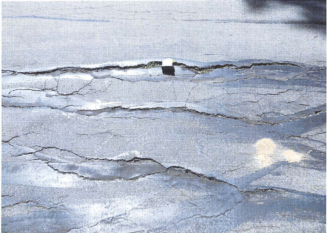
Photo 5: View of asphalt cracking in Vista Drive suggestive of landslide activity.
