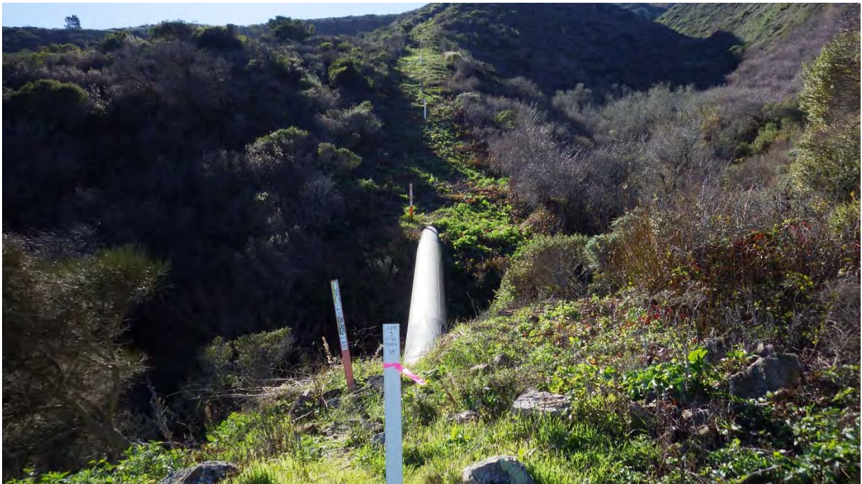
Photo D3 – Upper Section D – Exposed PG&E Gas Line
