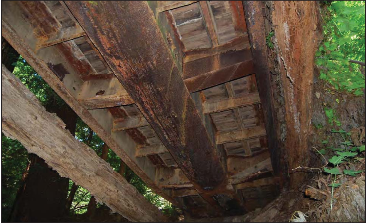
Figure 13: Soda Gulch Bridge, non-redundant main box girder with stringers, exterior girder and floor beams
